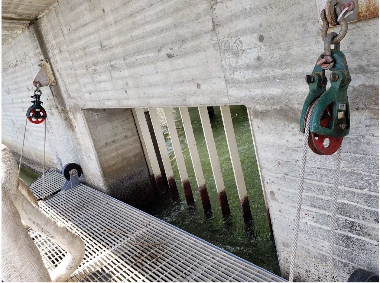
Floating and slide in trash racks before exclusion installed.
